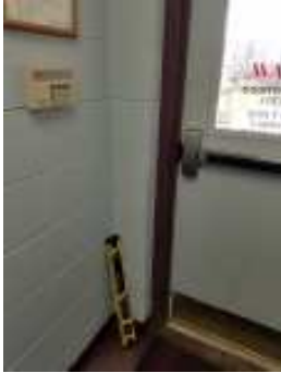
Finding #97, Additional Finding Photos
