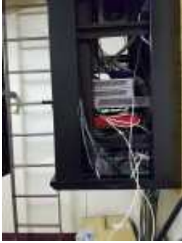
Finding #83, Additional Finding Photos
